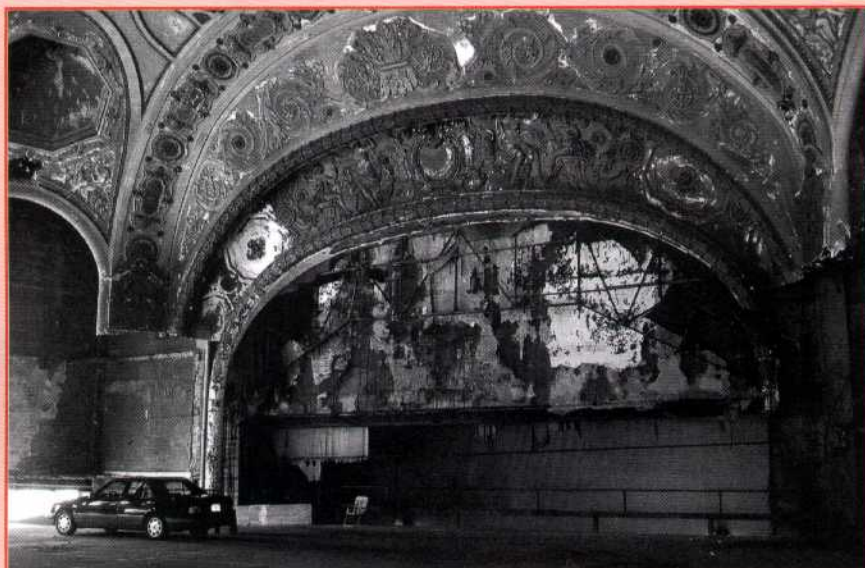
Figure No. 1: Michigan Building theatre interior at second level. Removal of the theatre seats and original partitions and decoration left the stark shell of the interior architecture. Currently used as a parking deck by office building tenants, it is unlikely that ongoing revitalization in downtown Detroit will return this theatre to its original use.
